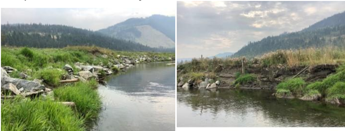
Failing enhancement documented in segment 9
